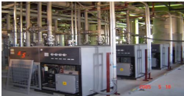
Clean Dry Air
